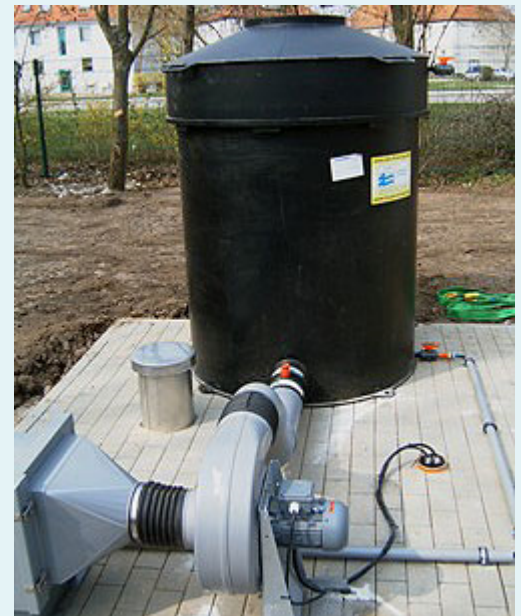
BEGA system for exhaust air from a pumping station
